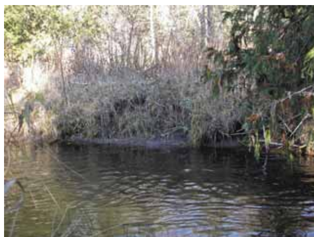
Photo 5: Slight erosion; re-grading and planting recommended
