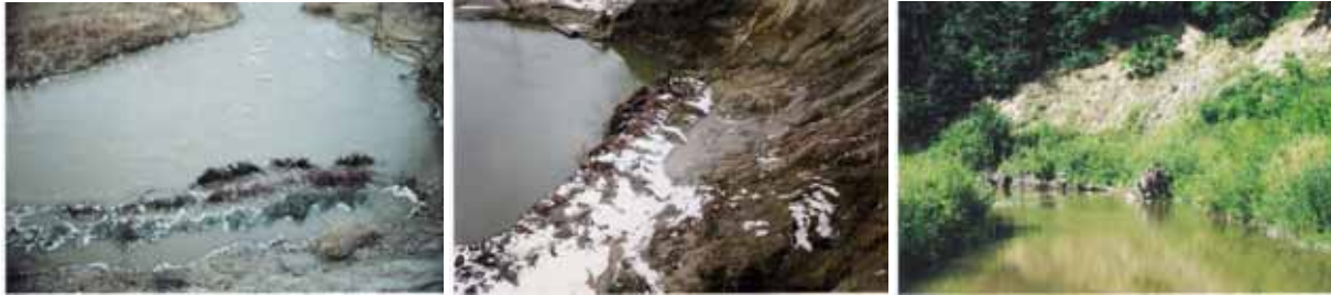
The series of photographs above show the progression of the East Humber structure.
